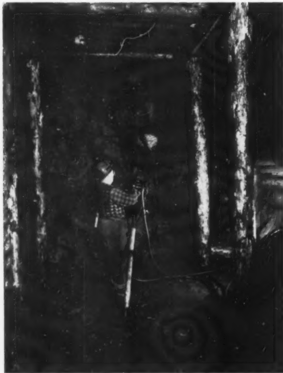
AIRLEGS are used to drill the rounds to advance cut across stope. No standard round is used because of the variable nature of the shattered ground. Great care is used to place and align lifter holes to grade so that the bottom breaks cleanly. This avoids any reblasting and popping the bottom to set stringers on line and grade and ensures a relatively smooth bottom for efficient slushing. Round is drilled, loaded, and shot to blast against log mat; not to damage stringers.
